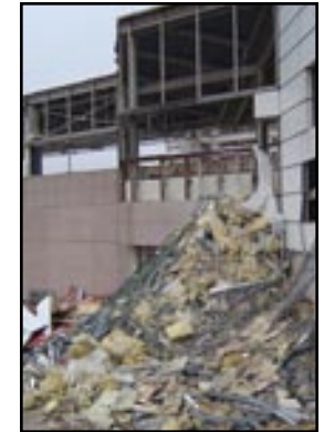
In the early stages of demolition, Terminal C interior building materials were removed and piled for sorting and recycling.
